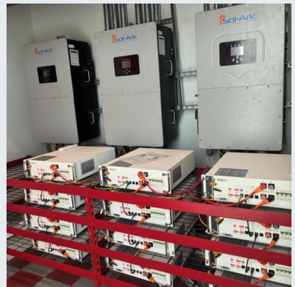
ESP-5K HL battery energy storage systems connected to Sol-Ark inverters
