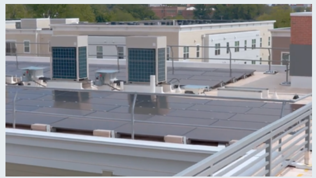
Rooftop solar on The Terraces at Park Heights
